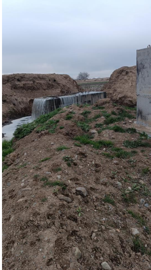
Figure 4 Observed wastewater discharge from collection pipelines in the project area (March 4, 2026)
